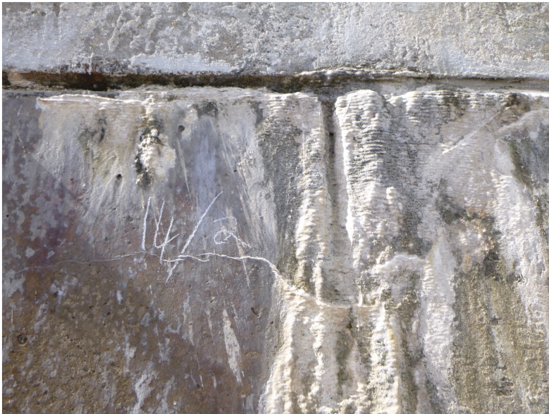
Photograph 5 – Defect 14-2 leakage through wall forming calcite dripstone
