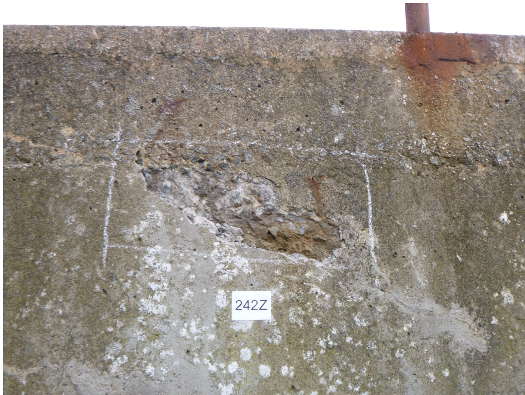
Photograph 4 – Defect 10-11 spalling parapet wall
