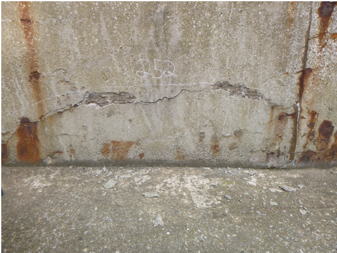
Photograph 3 – Defect 4-13 corrosion damage to parapet wall
