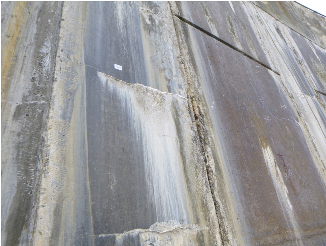
Photograph 9 – Defect 33-8 cracking and calcite staining
