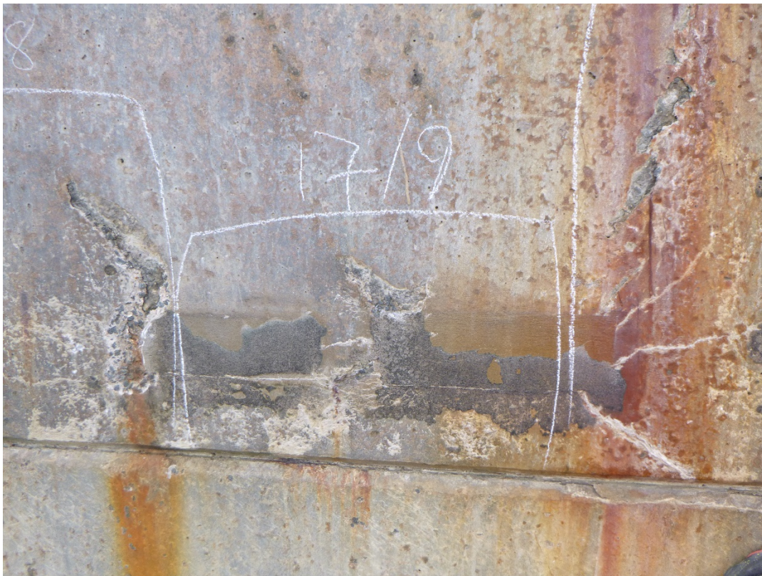
Photograph 6 – Defect 17-9 area of delamination and corrosion staining
