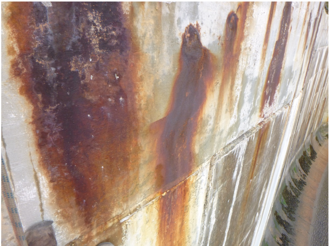
Photograph 10 – Defect 42-3 corrosion staining to panel
